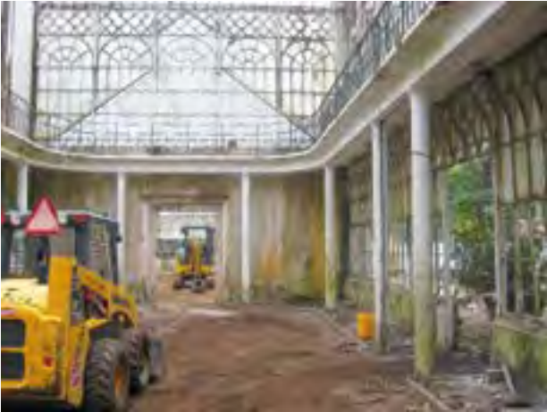
4. Image taken during the demolition of the gallery in reinforced concrete of the central body of the Greenhouses of the Botanical Garden.
