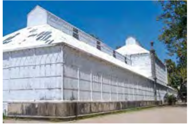
3. Exterior of greenhouses using the whitening process, prior to the recent restoration work.
