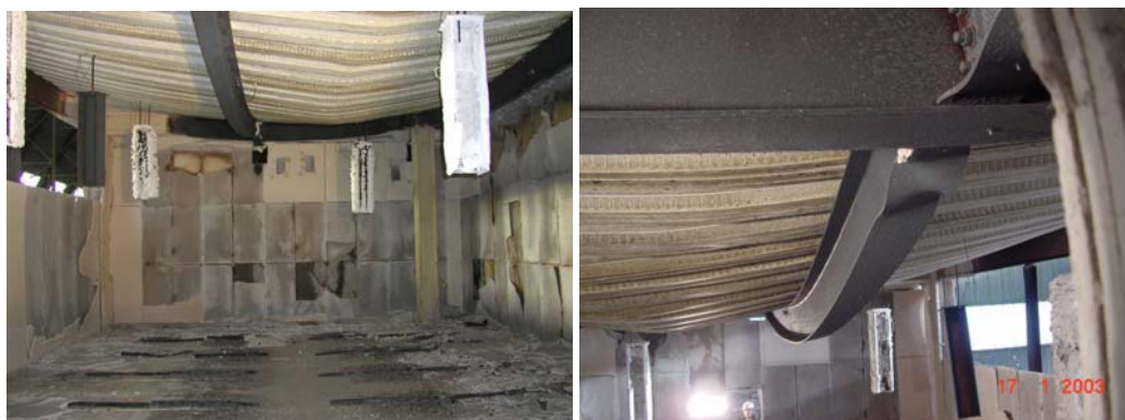
Fig 7 Compartment after fire, residual deformation 925 mm, no local collapse of structure
